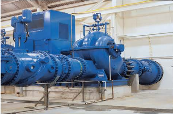
Patterson Horizontal Split Case Pump Station.
