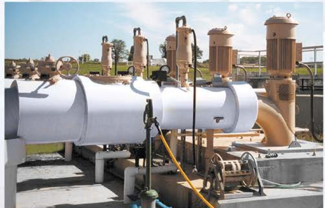
PVT Vertical Turbine Pump Station.
