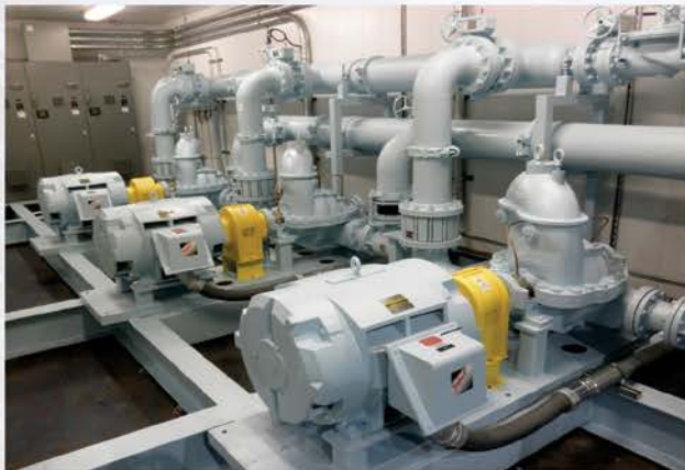
Industrial Pump Station Systems
