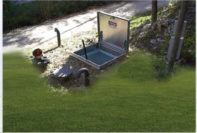
Entry Hatch and Ventilation Tube
