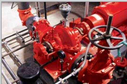
Horizontal Split Case Fire Pump with electric motor.
